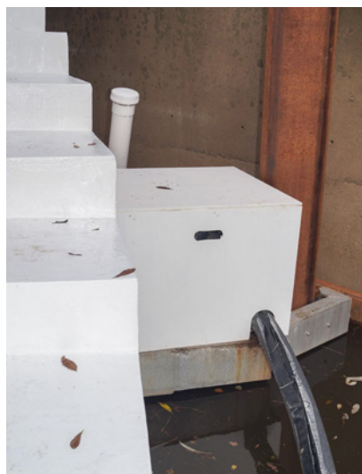
The Saniflo 110 is installed in a box adjacent to the house and floats up and down with the house as the tide moves.
