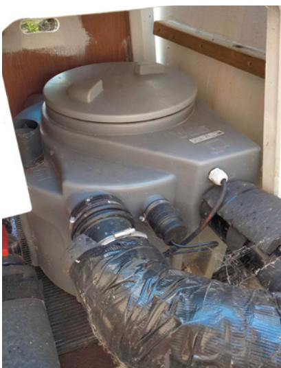
The Saniflo 110 takes the waste from the internal pumps and discharges it through small bore pipework up the hill to the mains drains.
